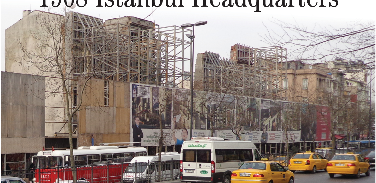
Sakız Ağacı today is sealed off for redevelopment. On the other side of the fence stand what used to be the Anarad Hughsouthoun School for Girls, the Surp Anna Catholic Orphanage, and the Mkhitarian Catholic School for Boys. (Photo: Varak Ketsemanian)
